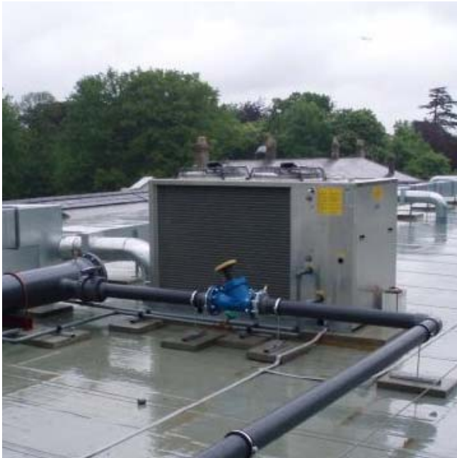
Low profile roof units installed at the prestigious 5 star Luton Hoo Hotel
