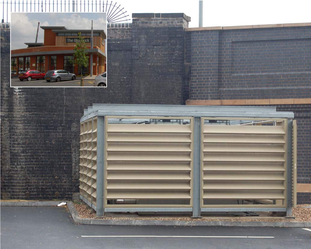
External units can be installed away from the main site if necessary as was the case at the Premier Inn Hotel, Wolverhampton.
